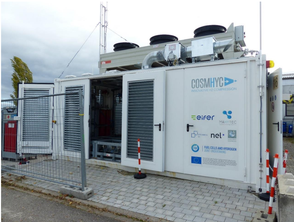
COSMHYC container at the site of Fraunhofer ICT (close to Karlsruhe, Germany) containing the metal hydride compressor and testing equipment
